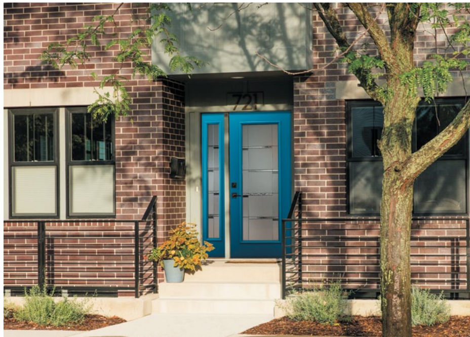
Door 89 CWK-NI Sidelight L150 CWK-NI AS, FB, MB, MGC, S, SB, TB
